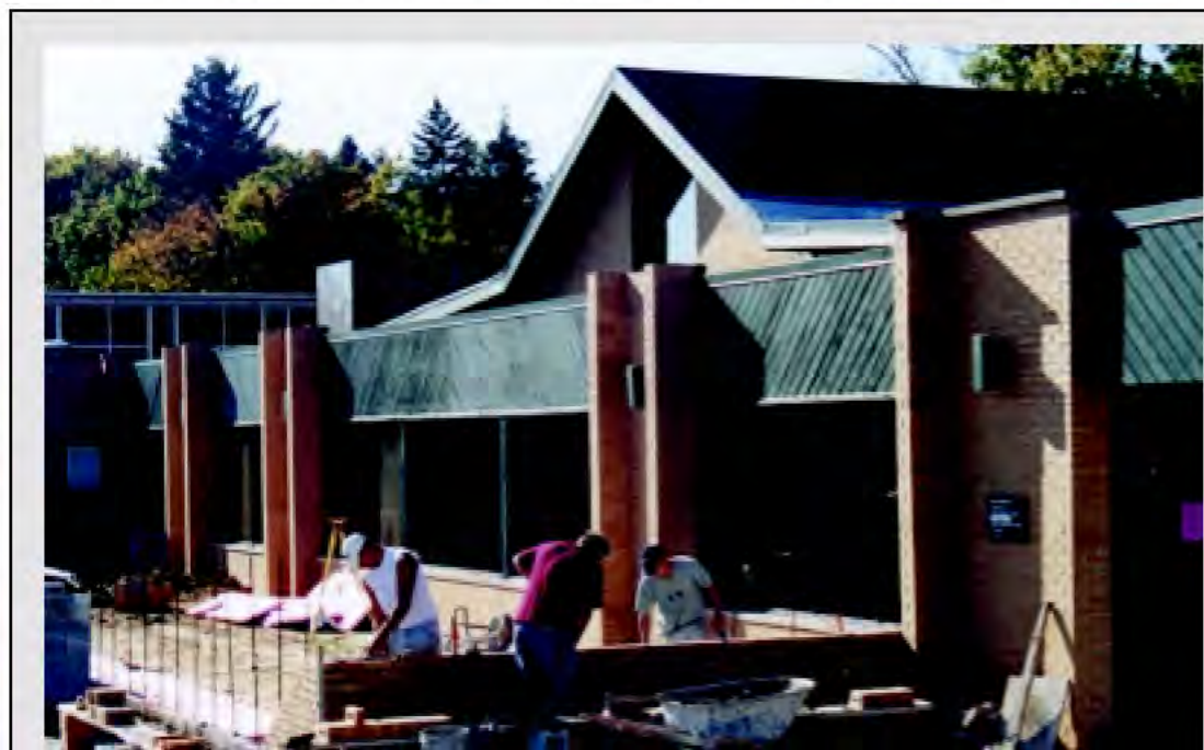
Construction on the Isom Atrium began shortly after the opening of the new academic year. The glass structure, attached to the Westside-Central Auditorium, will provide additional social space for the campus community and will house the Solid Rock Cafe. Full occupancy of the facility is expected by the end of the semester. Further details will appear in the next issue of the North Star .
