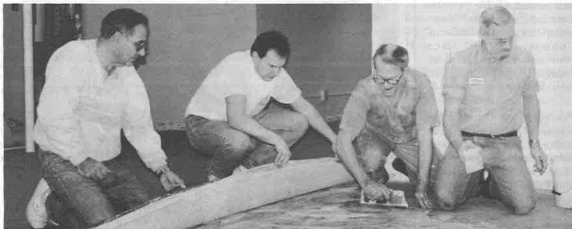
Volunteers Richard Haddad, Toby Osburn, and Charlie Tutor assist DuWayne Rathbun with the installation of new carpeting in the reference room of the Muirhead Library.
